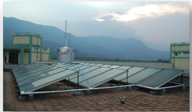
Solar Water Heater- Boys Hostel
