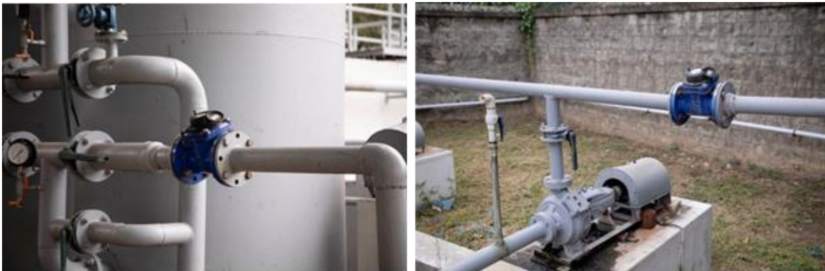
Flow Meters at the Filter Unit of Treatment Plant to measure the Treated Water
