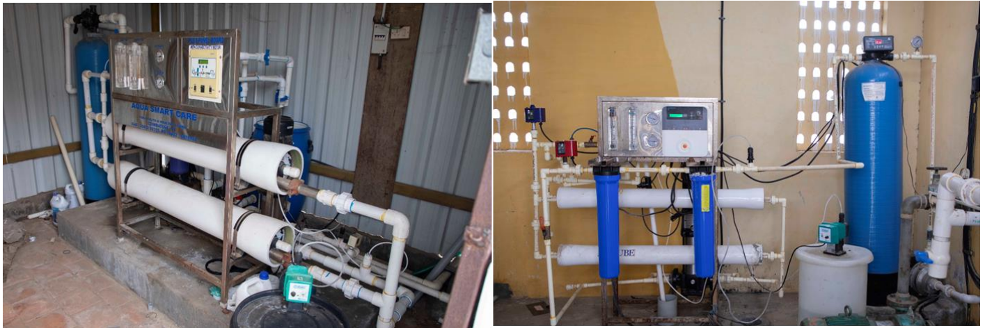
R.O Treated Water – For drinking and cooking
