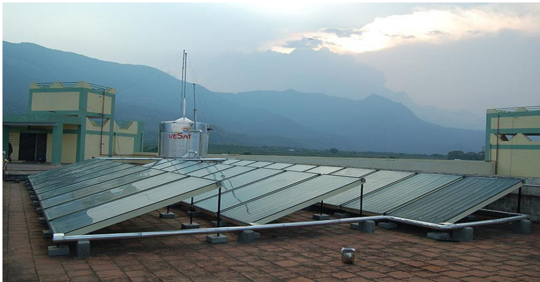
Solar Water Heating system in Student Residence
