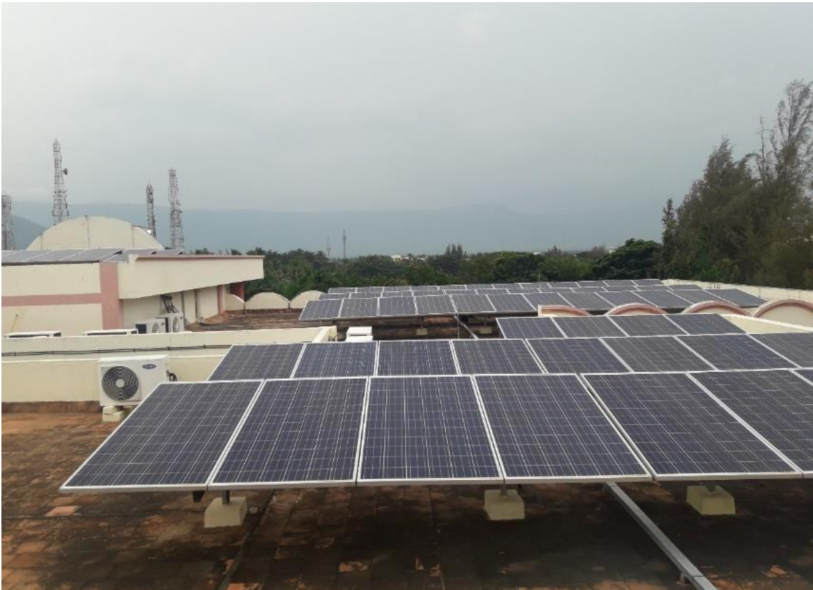
Solar Power Plant in Admin Block
