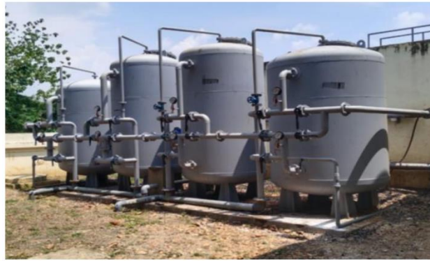
Air compressors and activated carbon tanks for de-odouring and clarification of treated water
